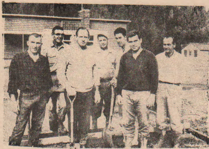
HARD WORKERS TAKE A BRIEF BREAK FROM POURING THE SLAB FOR THE NEW GAME COURT AT THE CHUGIAK SCHOOL. (left to right) DICK KERBOW, WALT PEASE, PAUL KERR, BILL BENYISH, AL TANNER, SAEMUS McGRADY AND BILL STEPHENS.
