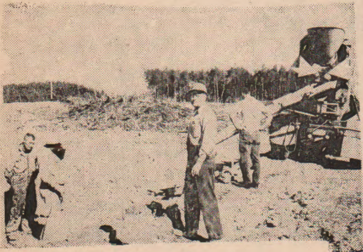
GENE EDMONDSON, FOREMAN FOR THE J.B. WARRACK COMPANY SUPERVISES THE POURING OF THE FOOTINGS FOR CHUGLAK HIGH SCHOOL.
