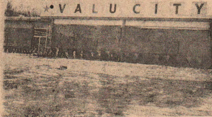
SHEETS OF PLYWOOD, HASTILY NAILED UP, COVER THE BROKEN WINDOWS OF THE VALU CITY STORE AT THE EAGLE RIVER SHOPPING CENTER. ONE OF THE MOST HEAVILY HIT OF THE LOCAL BUILDINGS BY LAST FRIDAY'S EARTHQUAKE.
