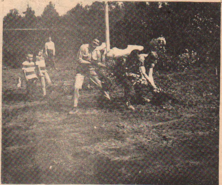
PULLING TOGETHER, THE CHUGIAK LIONS WORK HARD AT CLEARING THE BRUSH FROM THE CAR-NIVAL GROUNDS.
