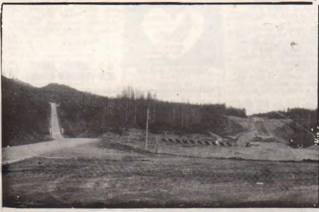
THE CUT IS COMPLETED. . . JUST WAITING FOR THE BRIDGE. THE APPROACH TO THE NEW PETERS CREEK BRIDGE IS FINISHED (right). THE PRESENT BRIDGE IS SEEN JUST A FEW HUNDRED YARDS UPSTREAM ON THE LEFT.
