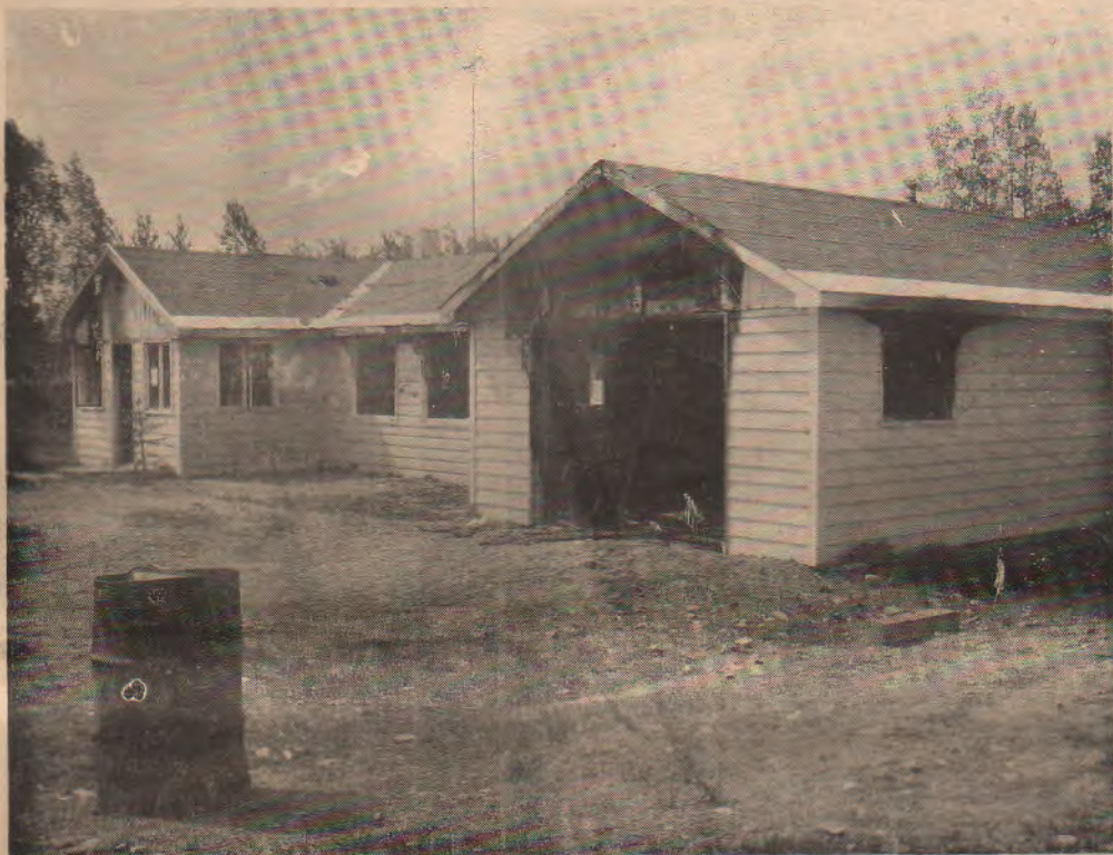
FIRE GUTTED RESIDENCE AT MILE 22 IS A GRIM REMINDER OF THE TRAGIC DEATH OF LOCAL WOMAN.
