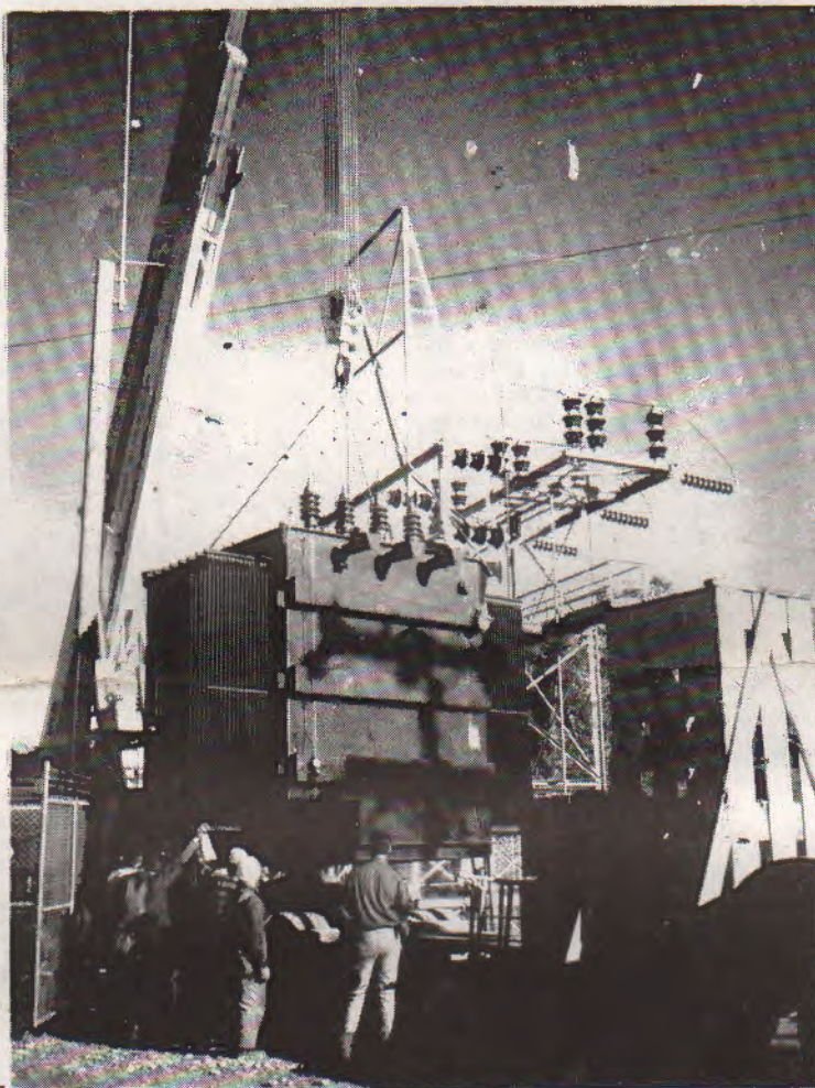
MEA CREWS HURRY TO REPLACE THE TRANSFORMER WHICH WAS HEAVILY DAMAGED BY FIRE AT THE PALMER SUBSTATION LAST SATURDAY NIGHT.
