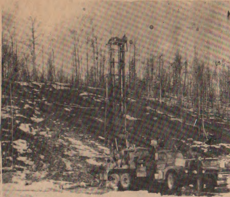
HATCH DRILLING RIG, AT WORK SINKING A WELL AT THE CHUGIAK ELEMENTARY.
