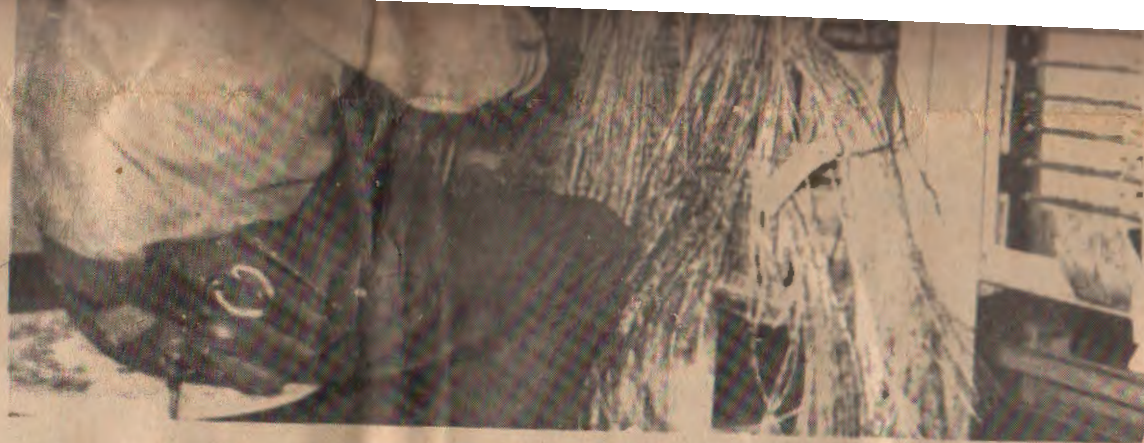
JOHN RIPLEY, TYEE FOREMAN INSTALLING A.N.I. EQUIPMENT AT CHUGIAK EXCHANGE (MTA Photo)
